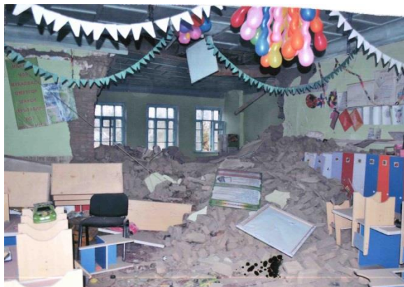
Classroom destroyed as a result of wall collapsed, ECD center in School # 31 in Panj district, Khatlon province, January 2015
